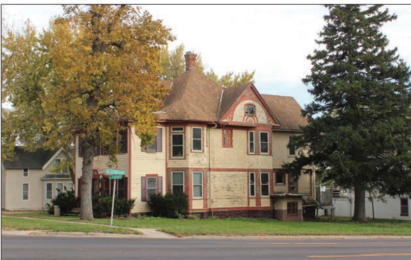
Property owners of this house on the corner of Lincoln Street and Highway 75 have been cited for numerous city code violations.
