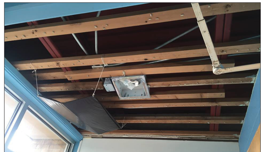
Necessary work at the Adrian library includes repairs to the ceiling and walls, flooring, light fixtures, ductwork, plumbing, electrical upgrades and more.
