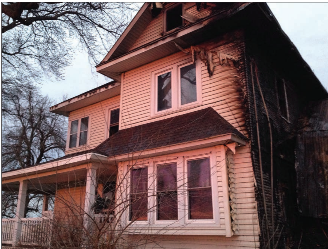
The Evers home on the south side of Kanaranzi was a total loss after the March 21 blaze.
