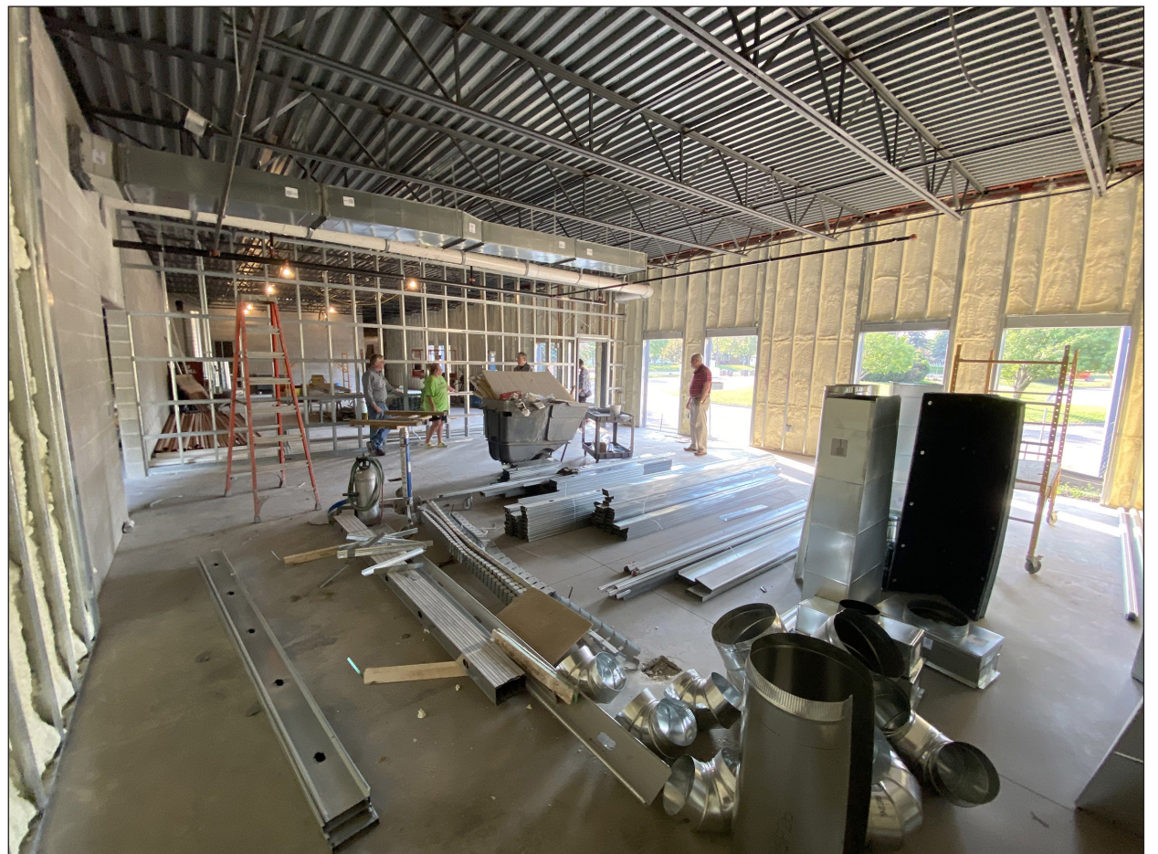
City council members tour the pool and fitness center construction this summer. This open area will become the new flat area for exercise classes and work-out videos.
