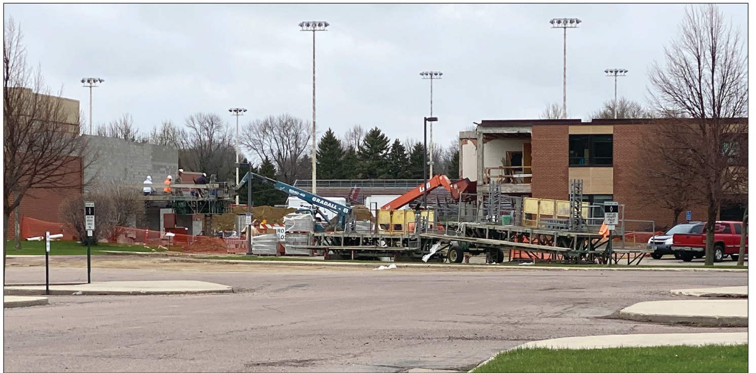
In 2020, workers from Gil Haugen Construction of Sioux Falls begin laying bricks for the new middle-high school commons and performing arts center that connects the middle-high school and the elementary buildings.
