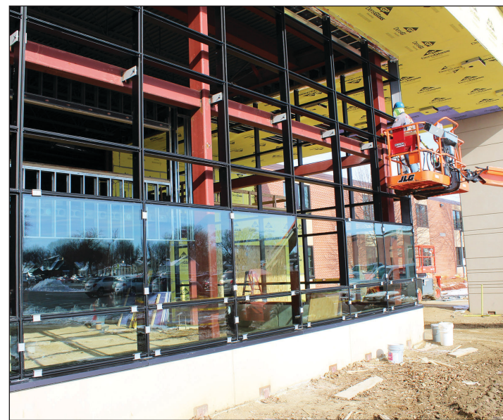
Workers install one of 63 windows to the new front entrance of the Luverne Middle-High School in November 2020. Entrance to the elementary, middle-high school, community education and the district office are now gained from the south side of the school campus along Dodge Street.
