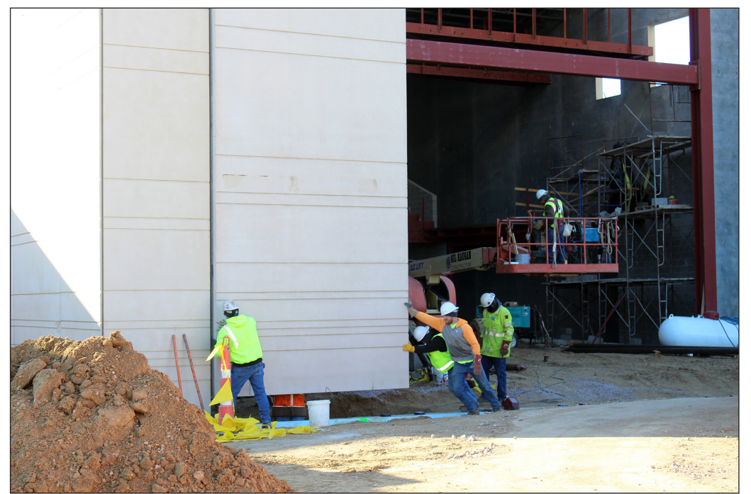
Gil Haugan Construction workers push the 56-foot-tall precast concrete panel in place.
