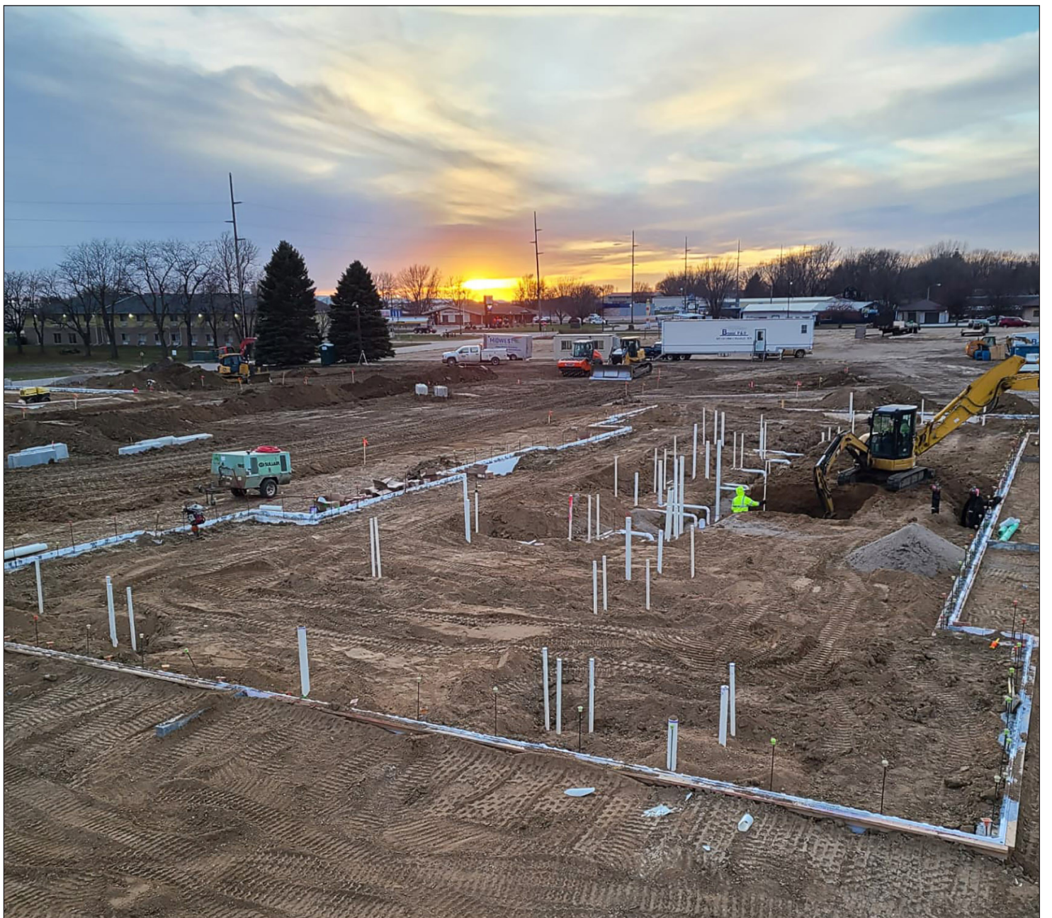
This photo, taken Friday evening from the Elevatex platform, shows foundations are poured, plumbing is roughed in, and prep work is underway for pouring concrete slabs next week, weather permitting. After that, framing will begin in January.
