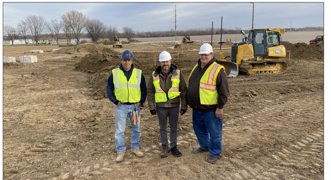
Luverne developer Don Jahnke of Midwest Sustainable Construction (left), investor Aaron Smith of Greensmith Builders and general contractor Mike Bourquin of Midwest Sustainable Construction meet at the construction site Friday afternoon along Hatting Street.
