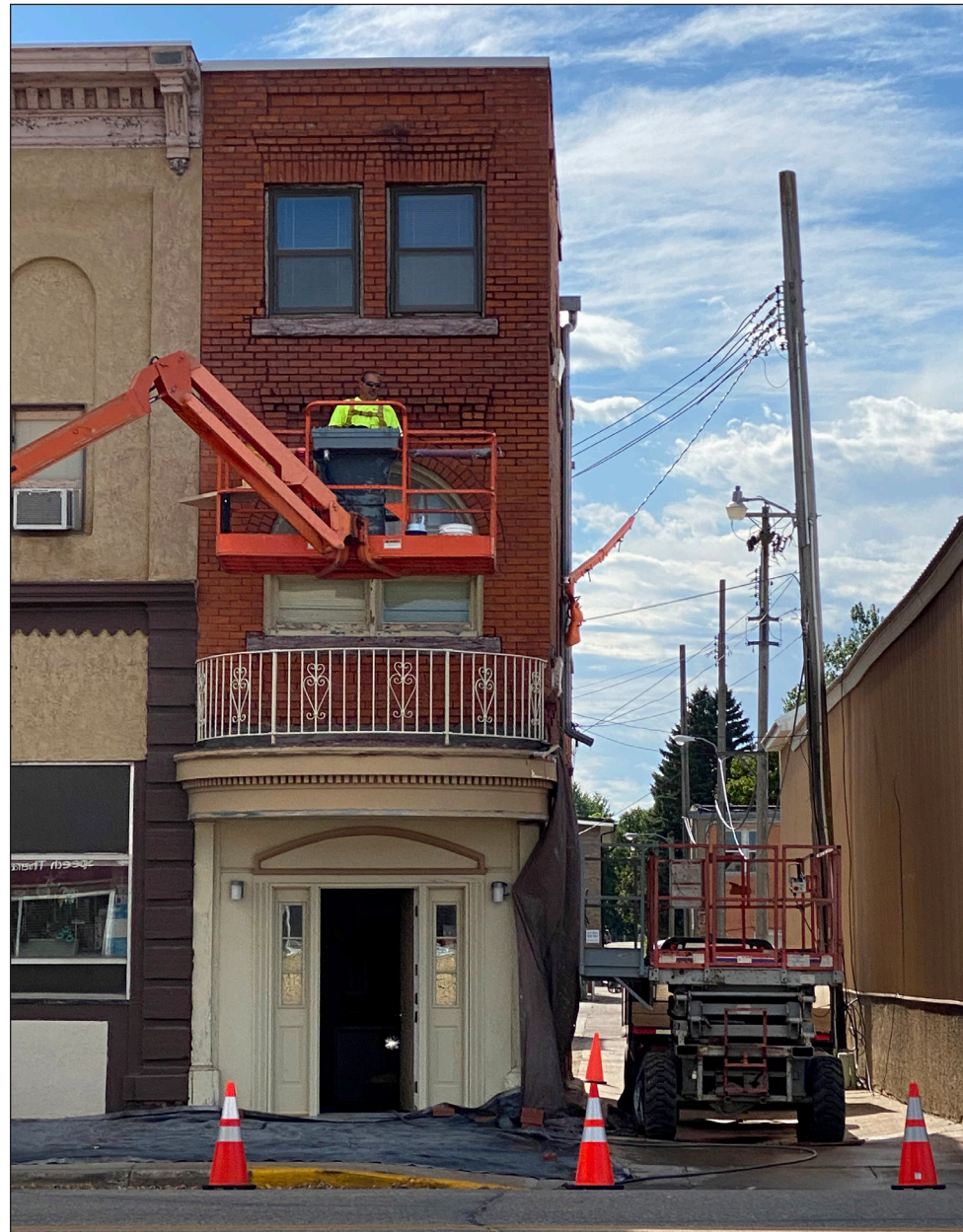
Contractors work on the facade improvement project for the Skinny Building on Cedar Avenue Tuesday, Aug. 11, as part of the city's historic facade improvement program.
