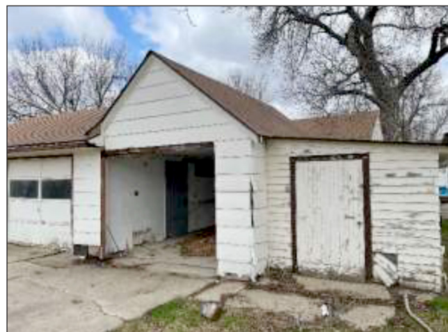
John Connell received a $3,000 demolition grant from the city to remove this property at 311 N. Oakley.
