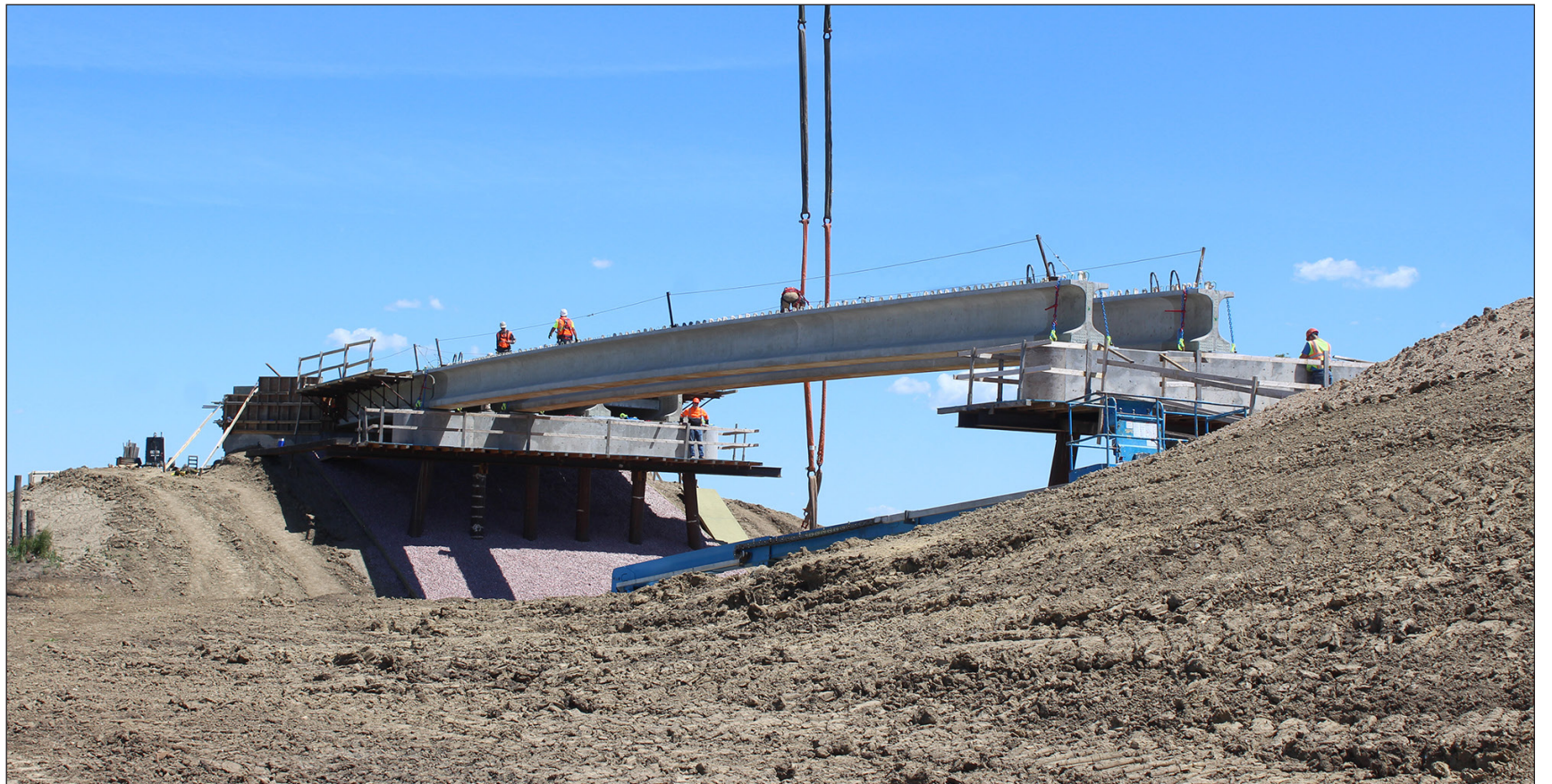
Straps are released from the second of four 93,000-pound, 106-foot-long concrete beams that were lifted into place by a crane Thursday morning, June 11, during construction on the County 52 bridge west of Beaver Creek. The new structure replaces the wooden bridge that burned in 2017.
