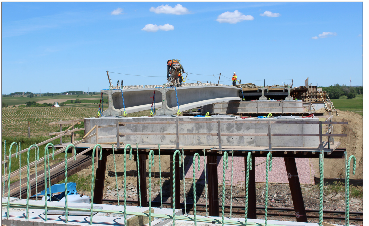
Balancing on the concrete bridge beams, Prahm Construction workers make measurements for the concrete decking that will cover the beams that stretch over the railroad.
