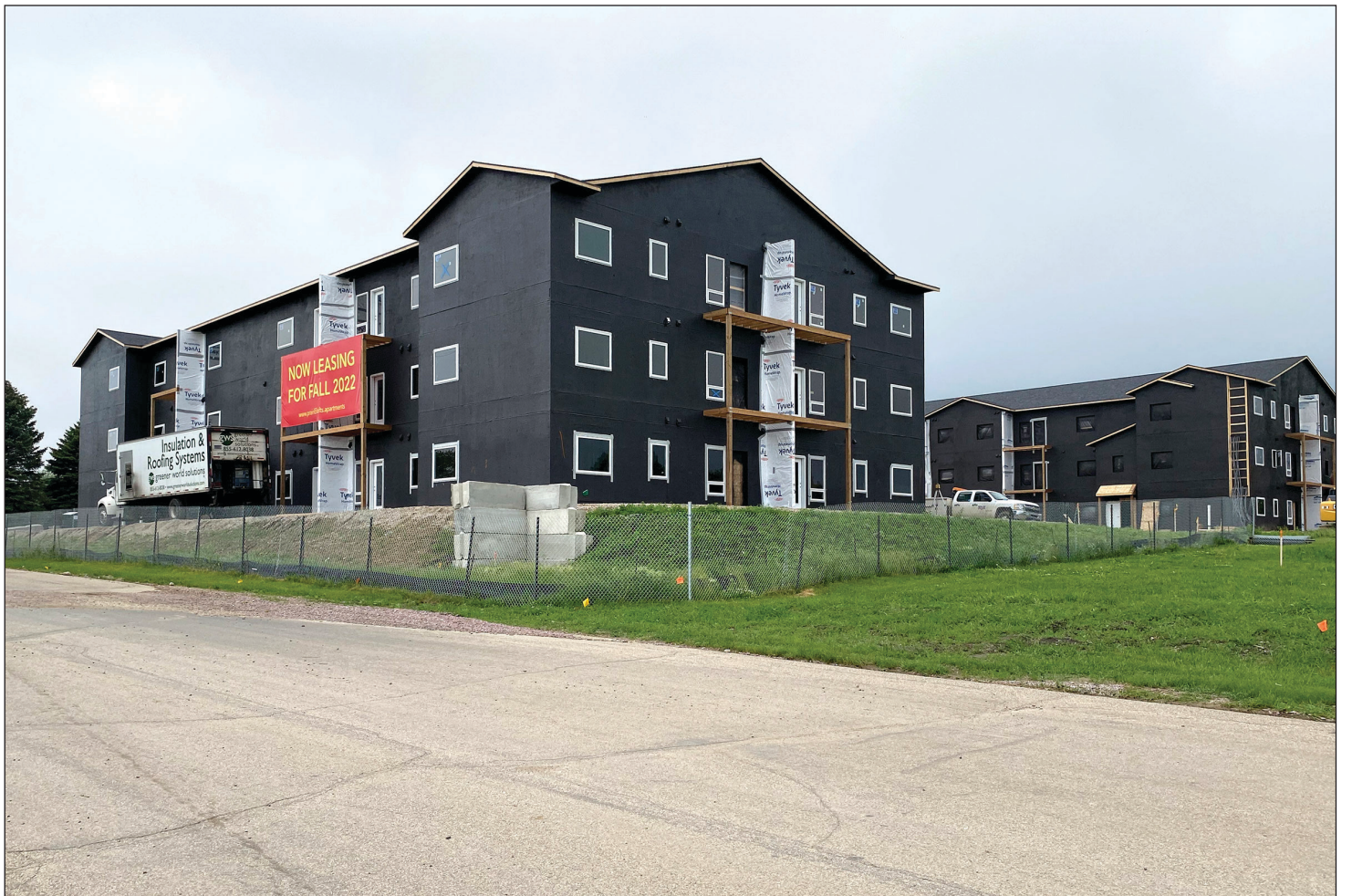
As construction continues on the Prairie Loft Apartment buildings in Luverne, the company is now advertising for fall lease arrangements. Two-bedroom, two-bathroom units of 896 square feet rent for $1,350 to $1,450. One-bedroom, one-bathroom units with 556 square feet rent for $900 to $1,050. Rental information is at GreenSmith.Builders. (Lori Sorenson photos)
