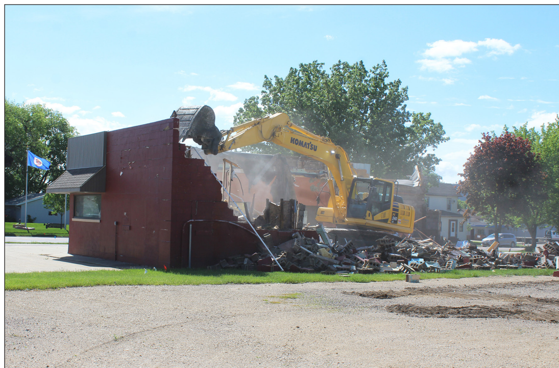
This is the back side of the former Remede building on June 1. It’s now a bare lot.
