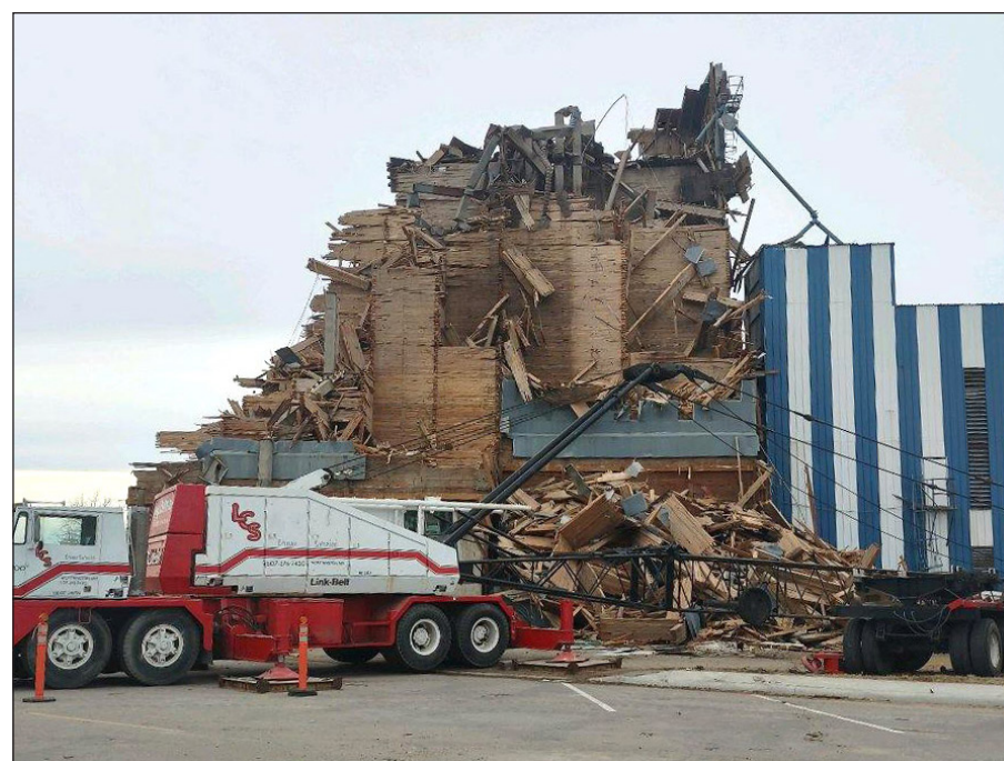
By the end of March, much of the former grain elevator had been reduced to a pile of rubbish. It was completely gone a month later.
