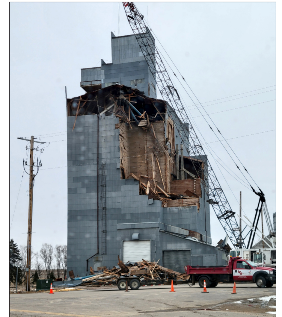
Beaver Creek maintenance supervisor Travis Helgeson shared this photo early in March when demolition started on the old wooden grain elevator.
