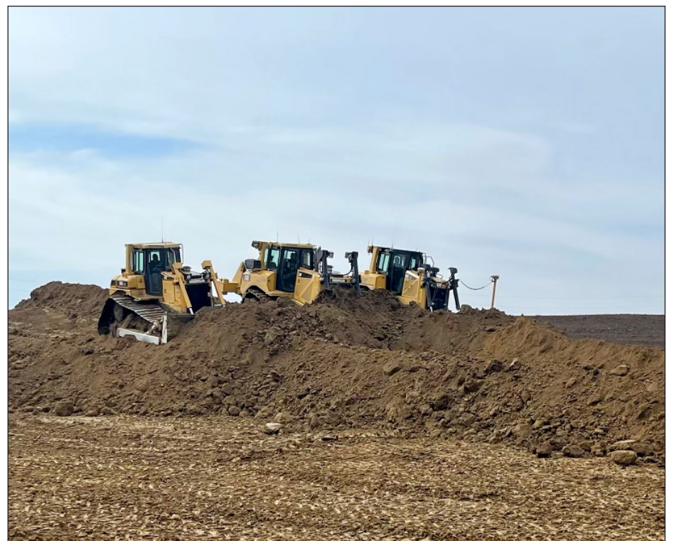
A trio of Henning Construction bulldozers team up to move dirt for Dakota Road in the industrial park ahead of the Lineage warehouse construction.
