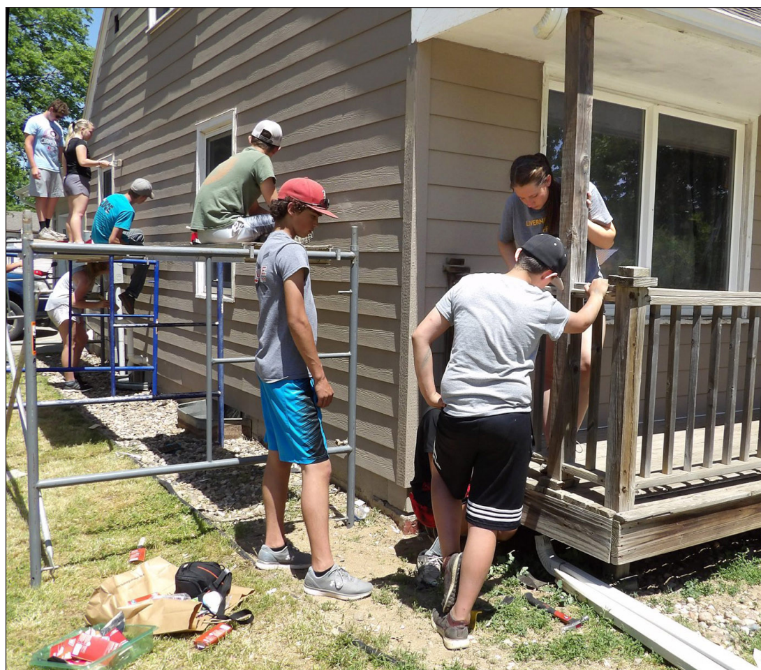
A group of teens with Rock the Edge Youth paint a house and repair a porch railing during the 2019 Service Over Self mission week in Rock County. The group is accepting project proposals for the 2021 mission June 21-25. See the Rock the Edge Facebook page for details.
