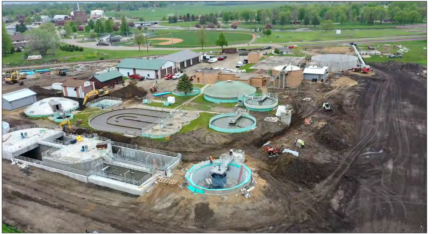
The city hired Luverne High School senior Cade Wenninger to photograph progress on the city wastewater treatment plant construction. Wenninger's Skygenix business started through CEO. The drone video is on the city's website.
