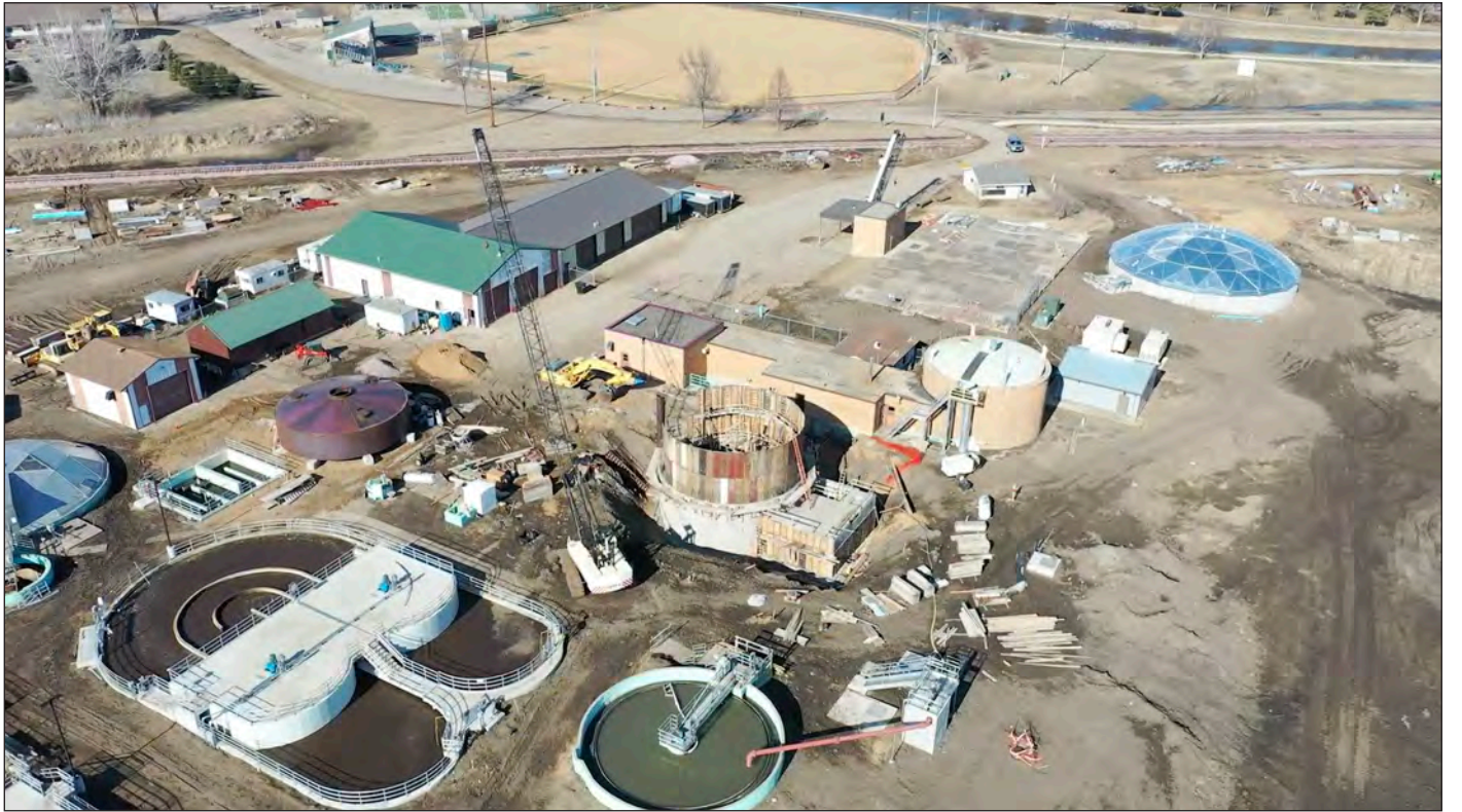
Drone images taken in May 2020 (top photo) and again in March (above and below) compare construction progress.
