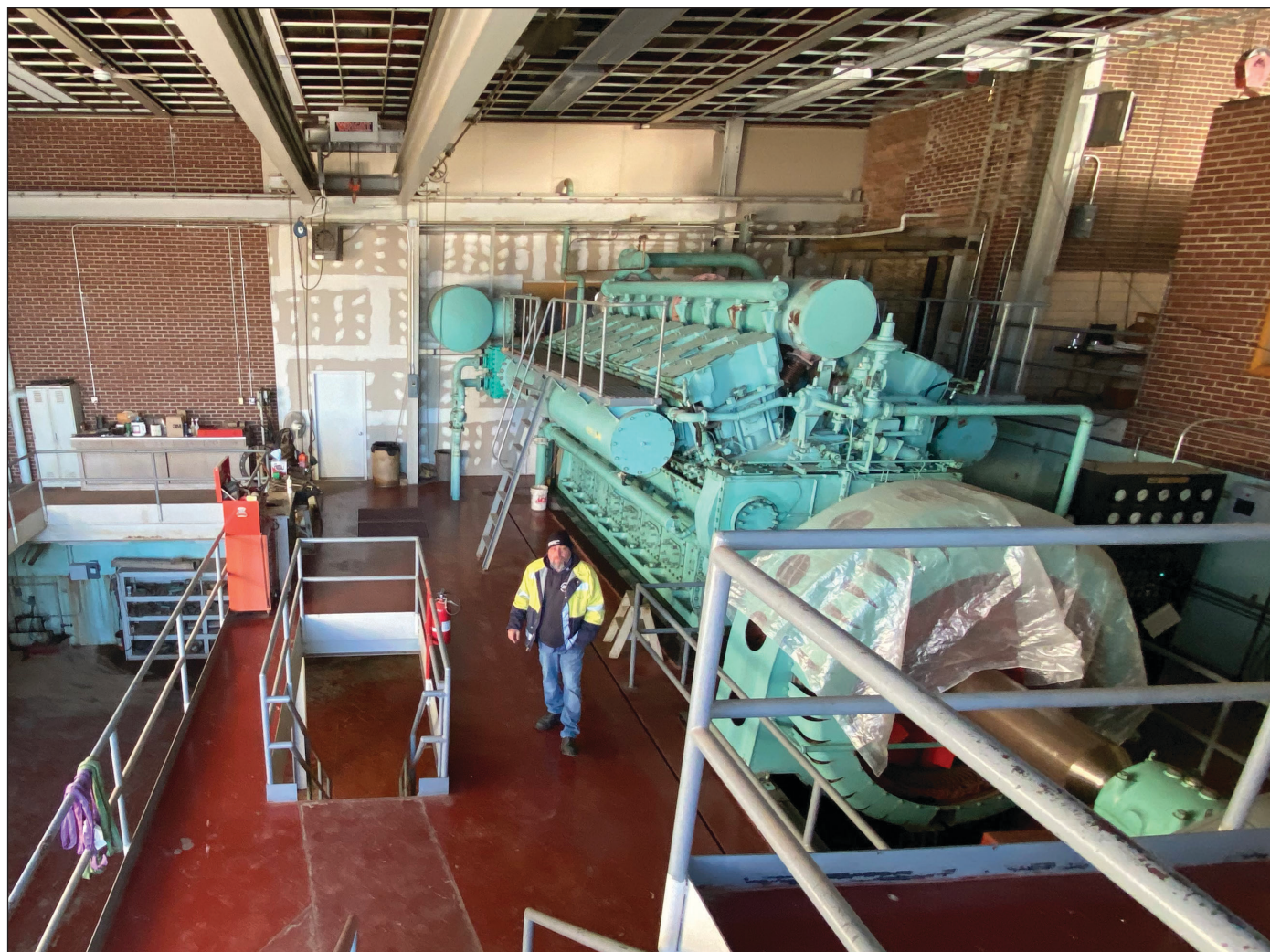
Lori Sorenson photo/0324 generator at power plant Dec. 16 photo
