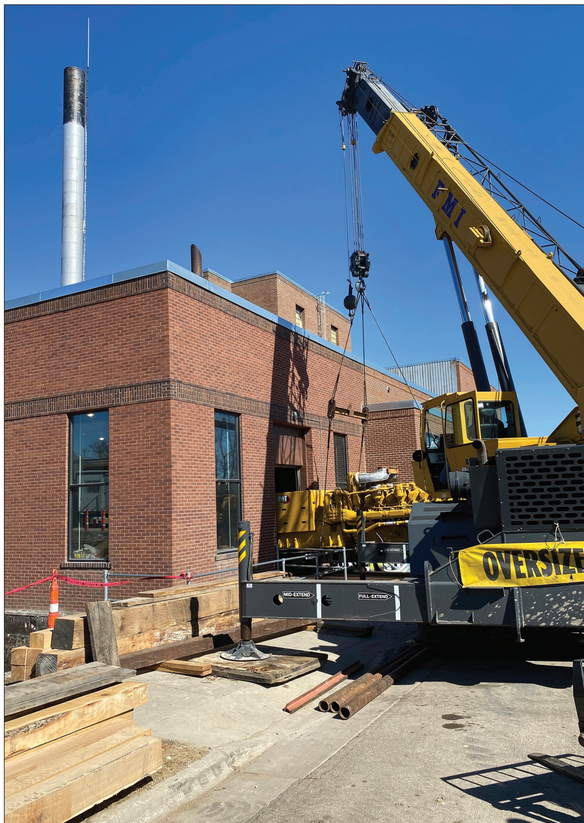
Lori Sorenson photos/0324 generator at power plant A crane eases a 50,000-pound Caterpillar generator into the Luverne power plant Tuesday afternoon on East Main Street. Another just like it was delivered Wednesday.
