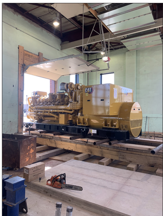
City electric supervisor Brian Remme shared this photo of a generator sliding into place on a series of pipes that were used to guide it into place Tuesday, March 15, in the power plant.
