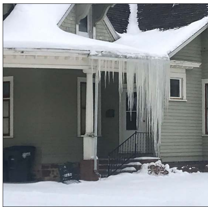
Lori Sorenson photo/0228 ice dam on north estey
