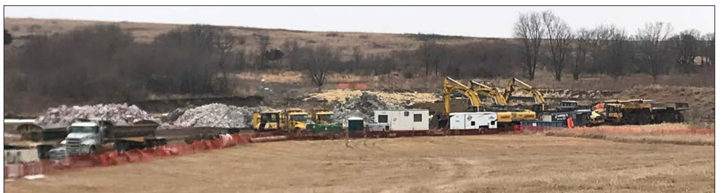
Heavy equipment lines up at the construction site of the Mounds Creek restoration during Christmas break. Lori Sorenson photos/0103 blue mounds state park creek restoration project
