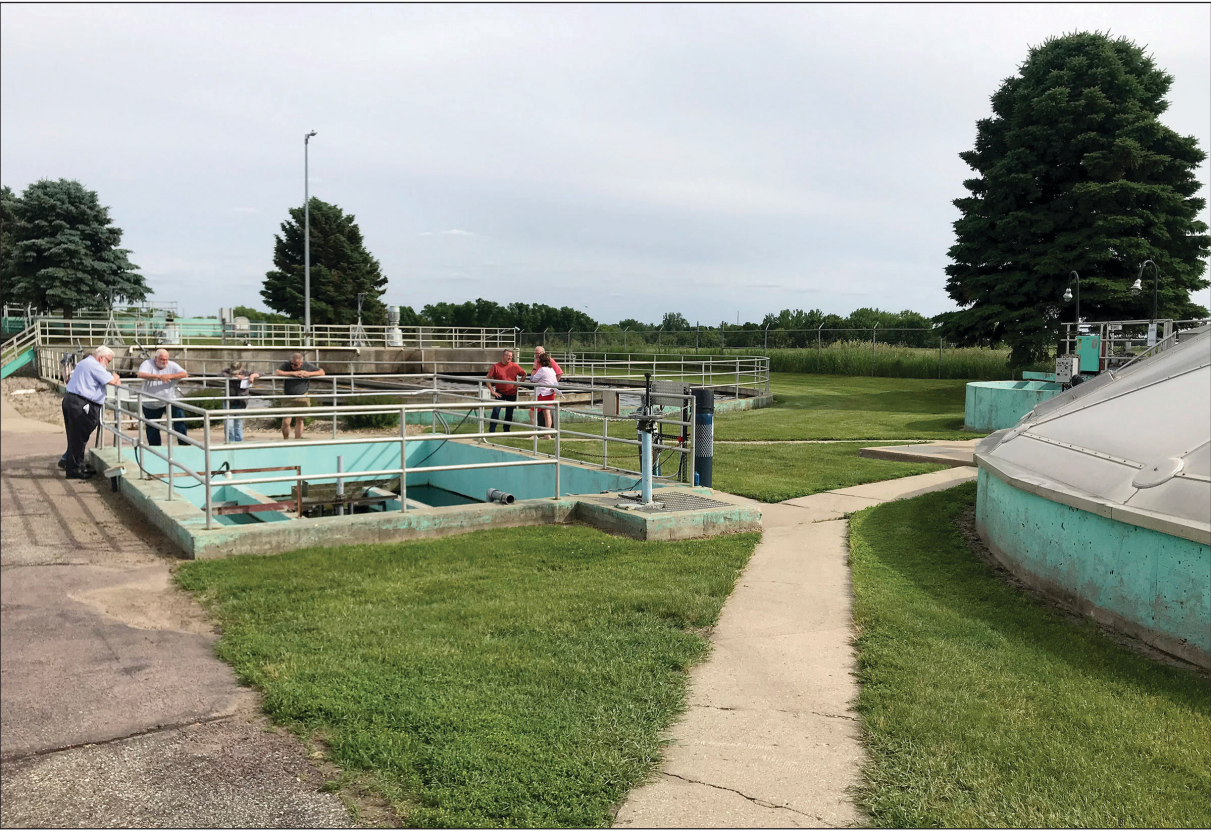
Lori Sorenson photo/0703 Wastewater Treatment Update
