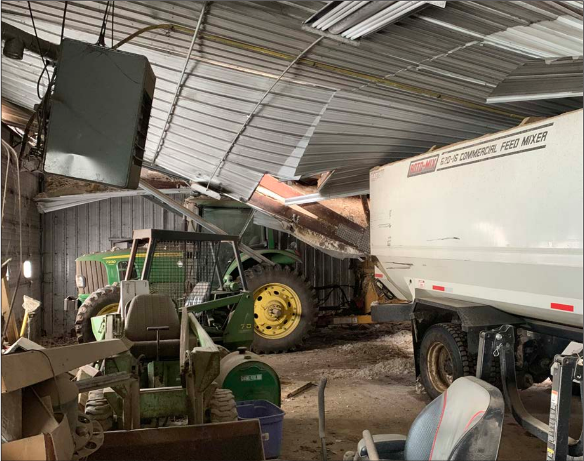
The 52-by-100-foot wood frame Morton building on the Ahrendt Bros. feedlot north of Luverne is a total loss, but equipment stored inside suffered only minor damage. (Submitted photos)
