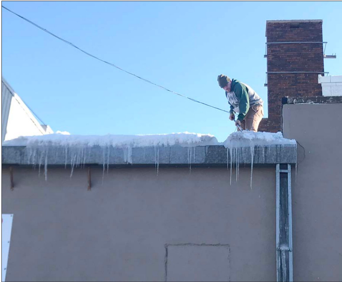
Lori Sorenson photo/0314 deboer ice dam
