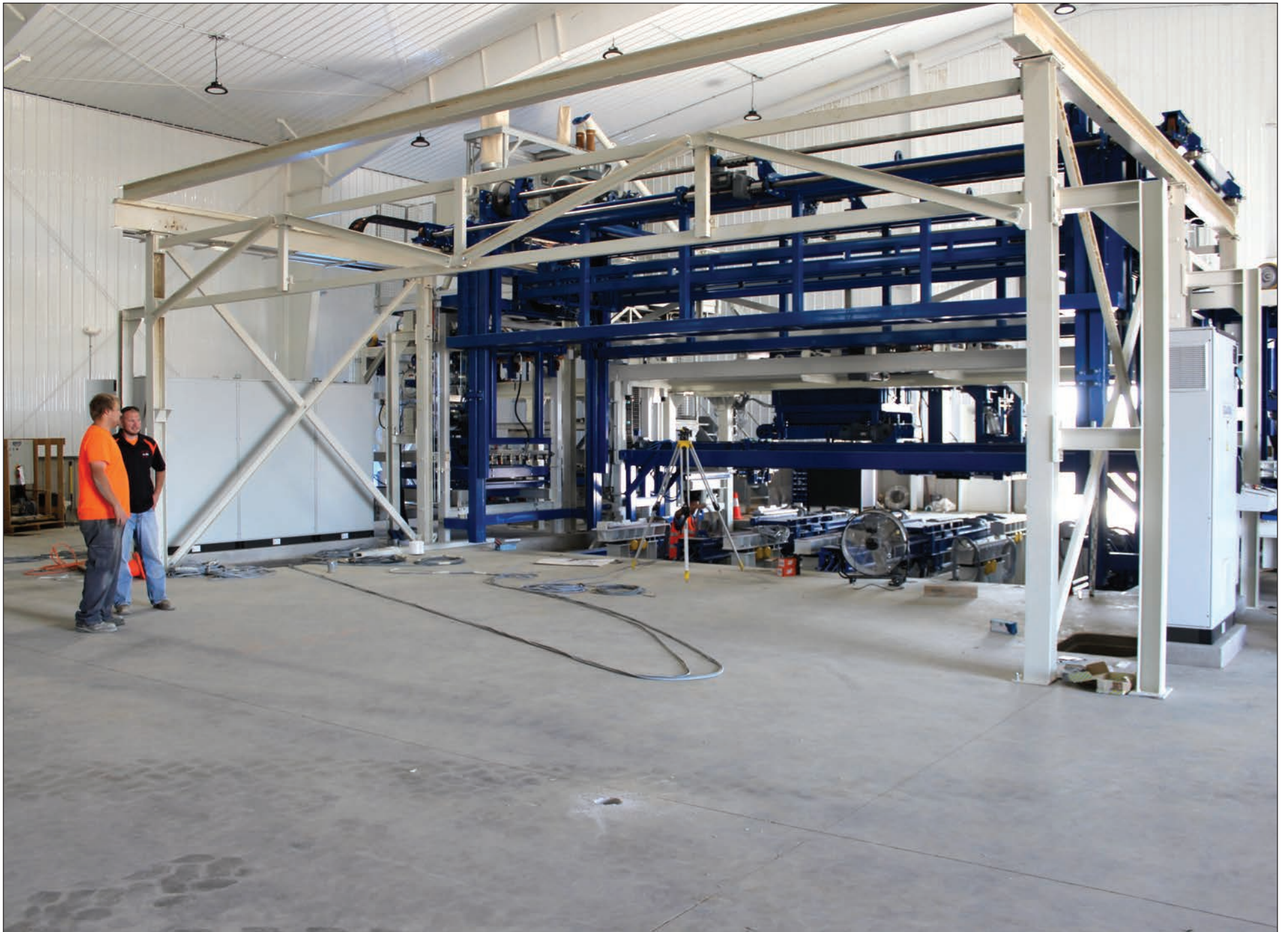
Mavis Fodness photo/Ag Tab Midwest Dry Cast AJ Pronk (left) with Buffalo Ridge Concrete and Midwest Dry Cast employee Alex Elgersma discuss the shuttle system that lifts the formed concrete products to the cure shed. The fully automated plant will blend the correct measures of aggregate, sand, cement powder mixture and water and press them onto one of two casting tables. Every 10 minutes the newly cast product is moved from the cast to one of multiple drying stations where steam cures the product to its final hardness.
